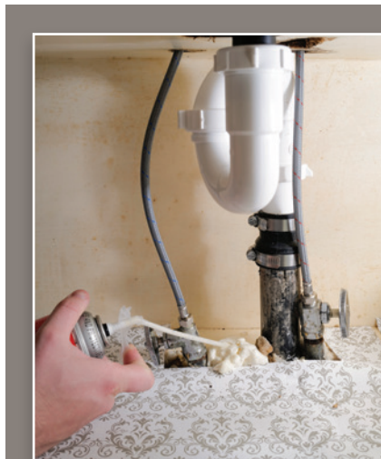
Spray foam seals gaps around pipes to prevent cold air from traveling up through those spaces, causing drafts and wasting energy.
